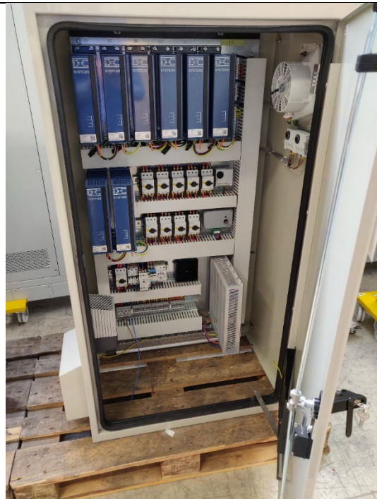
Outdoor substation for public lighting
