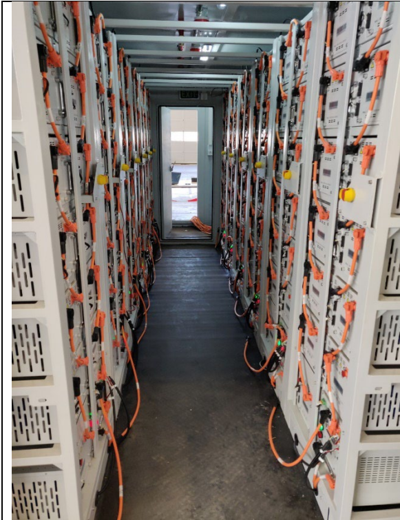
Distributed batteries system
